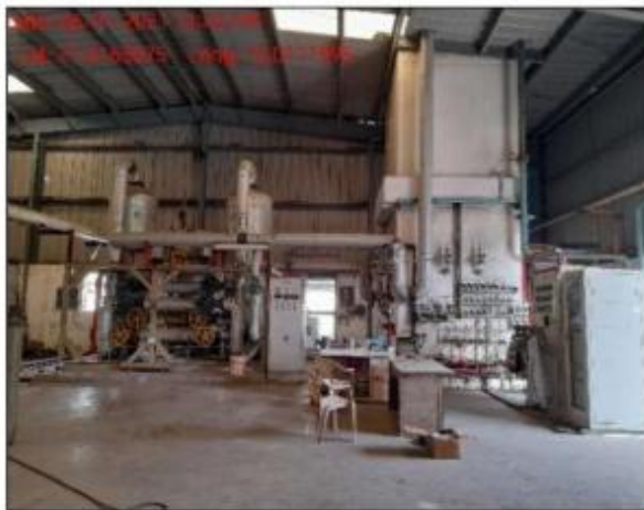
Critical Machines for Production
