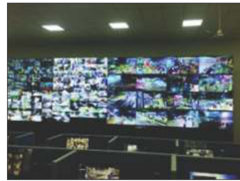
A glimpse of CCTV system installed at Still Tirumala Tirupati Devasthanam
